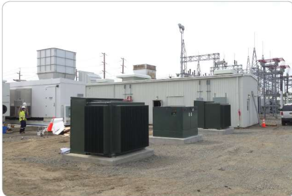
MULTI-STAGE FLYWHEEL/BATTERY ENERGY STORAGE SYSTEM Anchorage, Alaska
