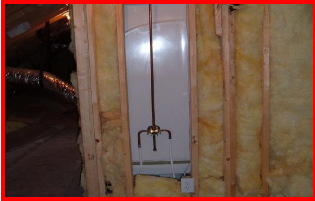
No air barrier installed prior to tub installation.
