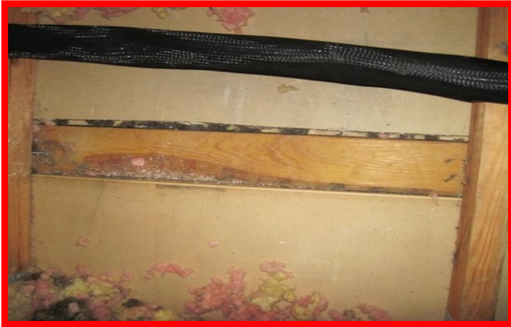
Top plate to drywall connection not sealed.
