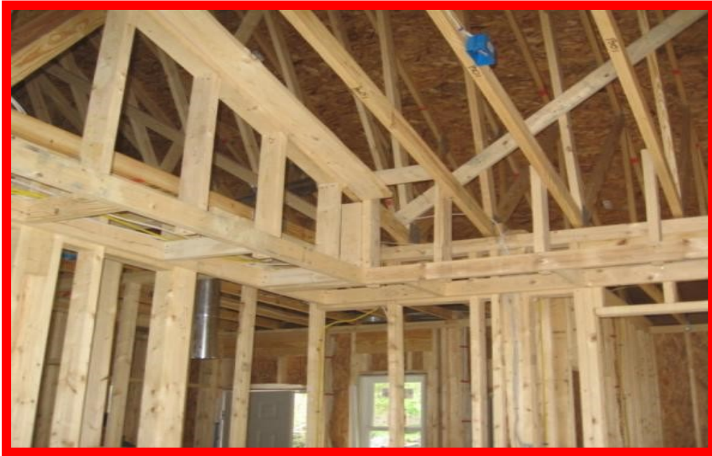
No air barrier is present between the dropped ceiling/soffit and the attic.
