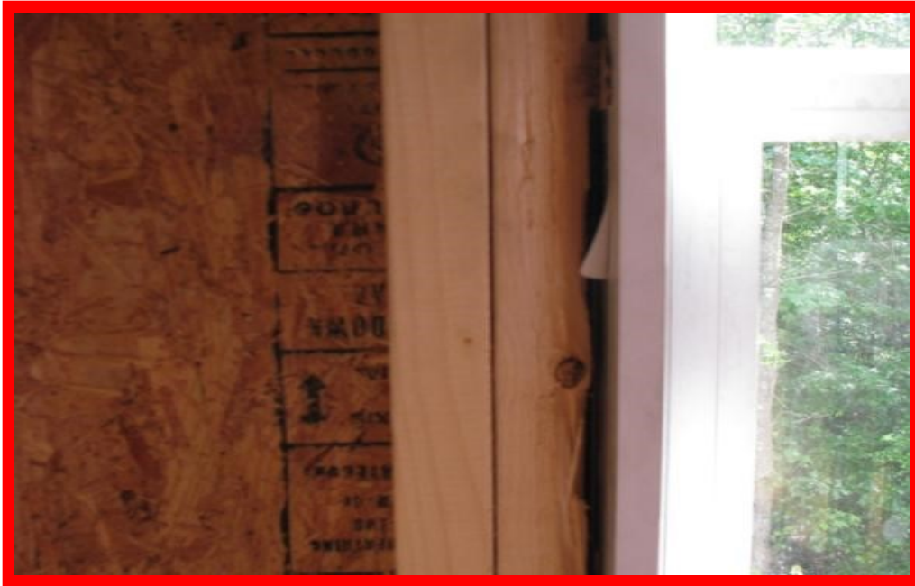
Rough opening around window not air sealed
