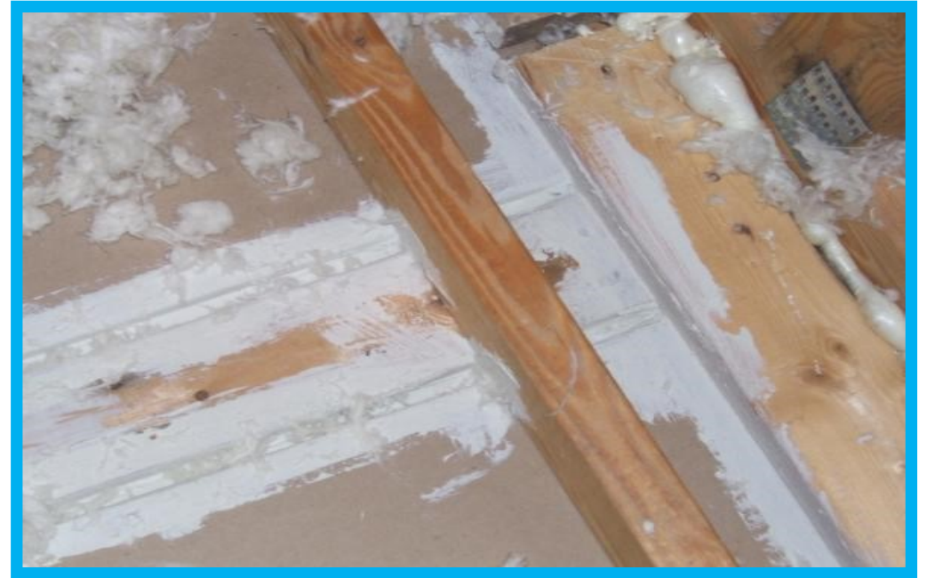
Top plate to drywall connection sealed from attic with caulk.
