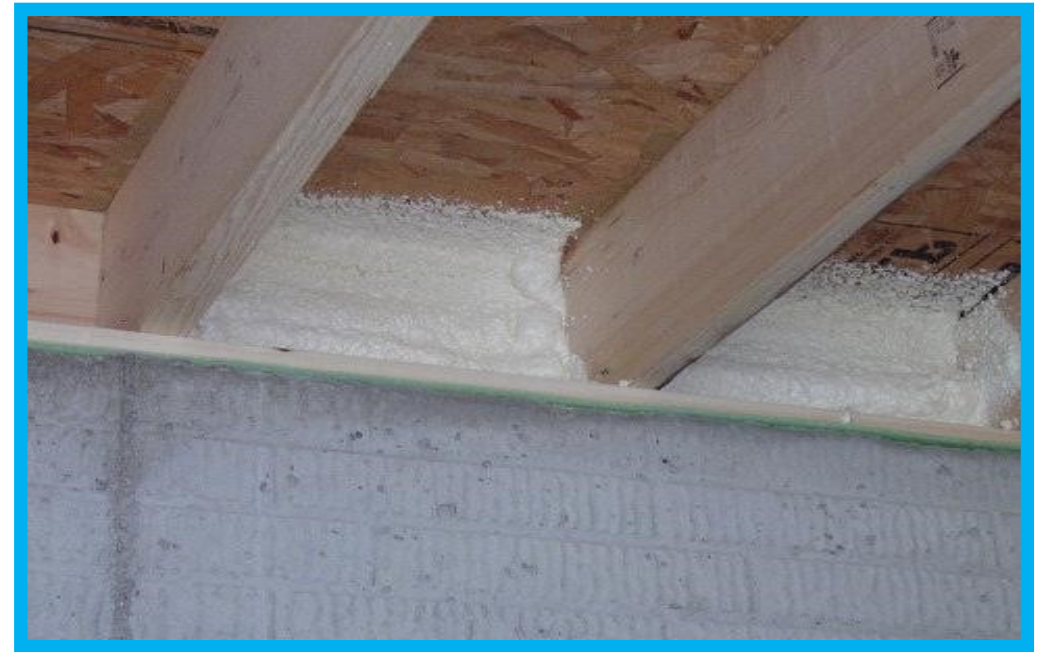
Band is properly insulated and sealed.
