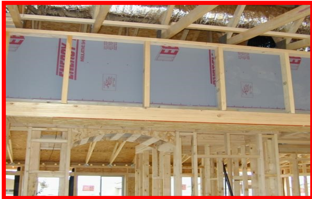
Backing not air sealed prior to insulation.
