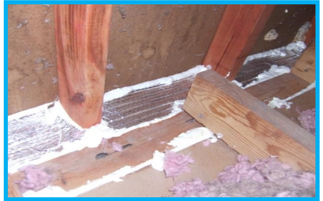
Blocking installed and air sealed instead of continuous top plate.
