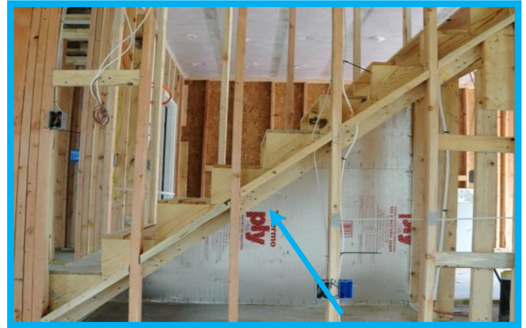
Air barrier installed under staircase. Picture taken from house looking into attached garage.
