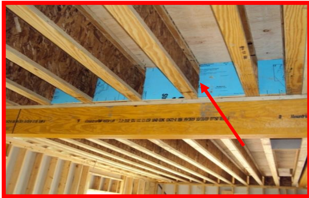
Gaps without insulation and not properly sealed.
