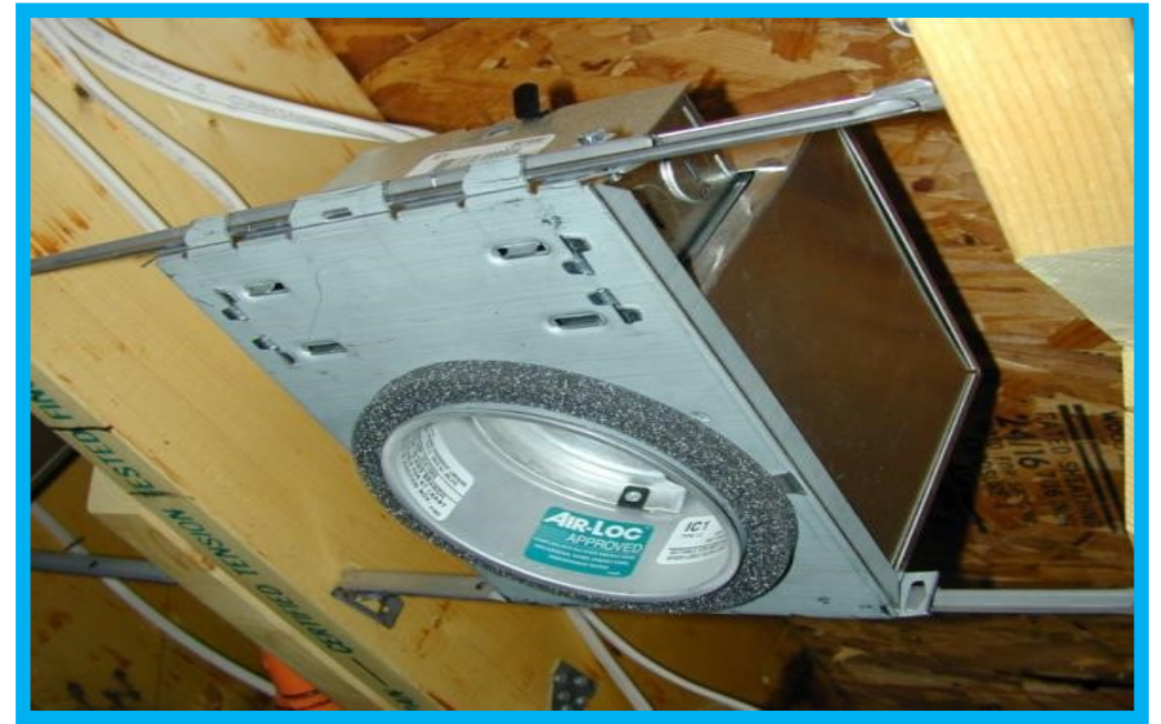
ICAT labeled recessed light with trim kit installed.
