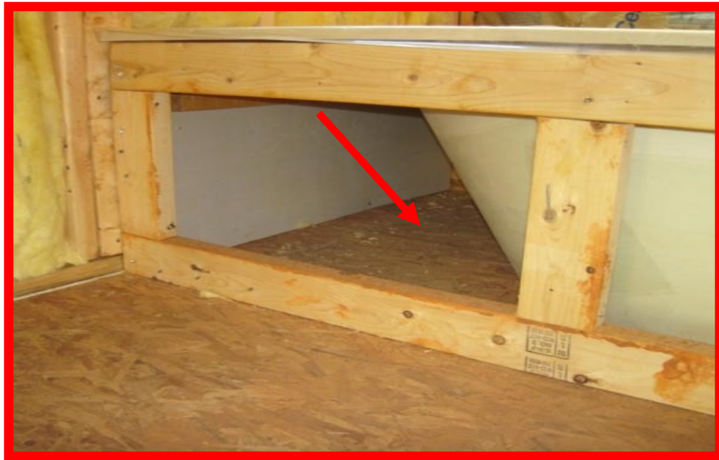
Air barrier not sealed.
