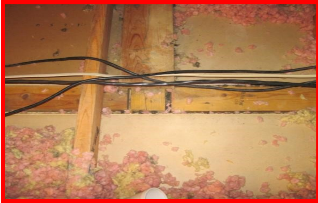
Top plate to drywall connection not sealed.
