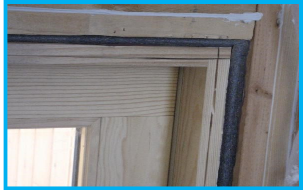
Rough opening around window has been filled with backer-rod to air seal.
