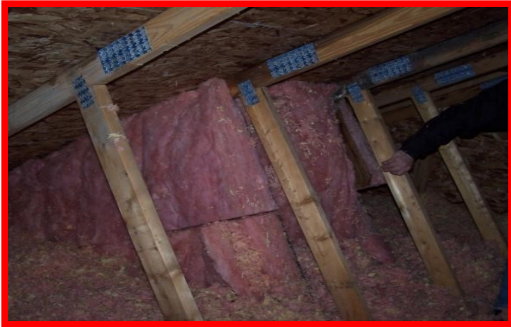
Rigid air barrier not installed to hold insulation in place.
