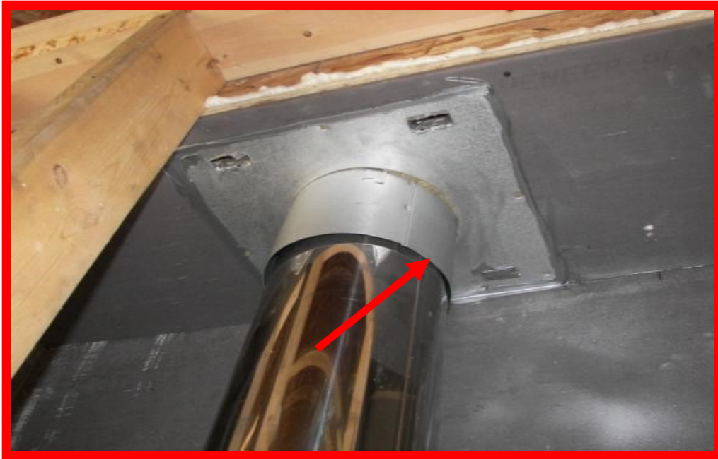
Vent sleeve not completely sealed.
